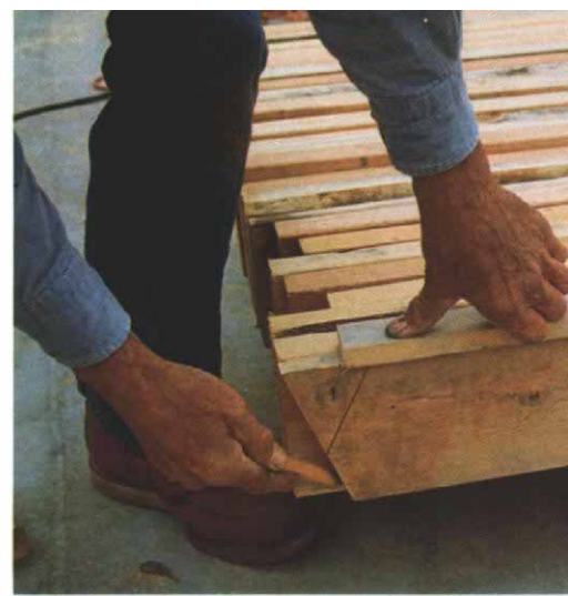
One way to lay out rafters is with a site-built rafter tee (photo above). The fence on top of the tee allows easy scribing of the ridge cuts and birds' mouths. When laid out this way, rafters are cut one at a time with a circular saw.
