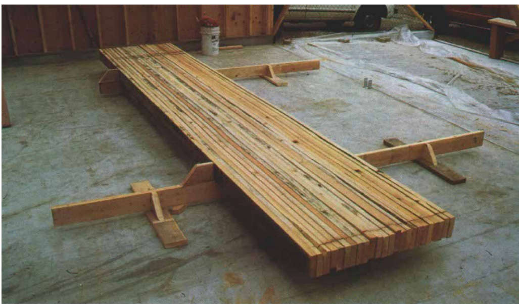
Piecoworkers typically build a pair of simple portable rafter horses (photo above). The horses allow them to stack rafters off the ground on edge so that they can mark and cut the rafters all at once.
